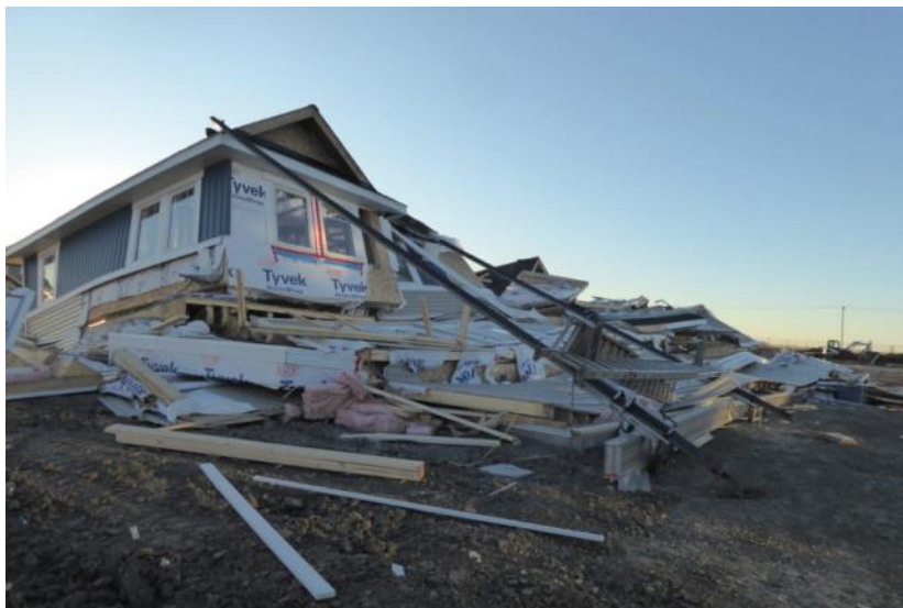
Partially constructed townhomes collapsed in Regina, Saskatchewan October 18, 2017 (Source: Kevin Martel, 980 CJME)
